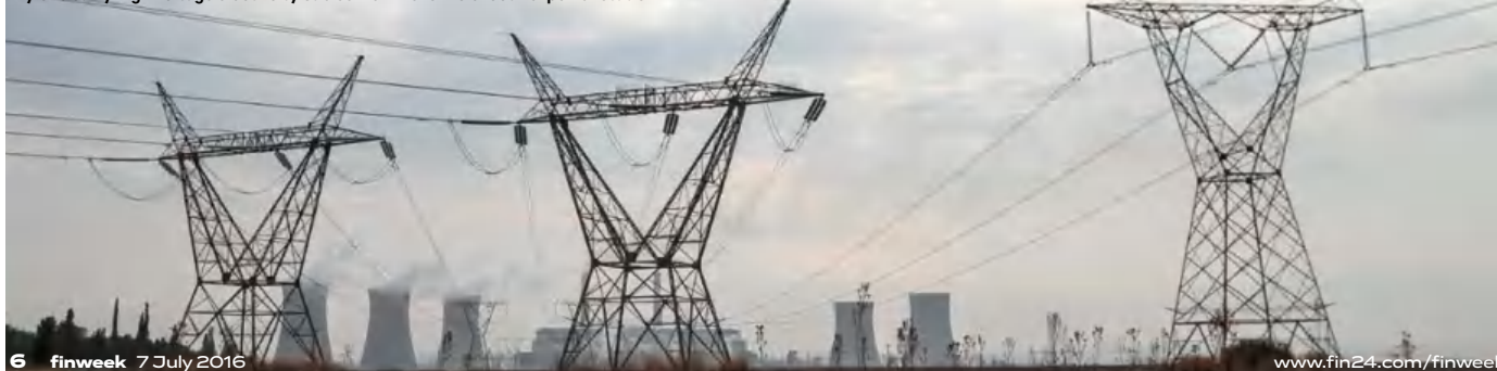
Pylons carry high voltage electricity cables from Eskom's Grootvlei power station.
